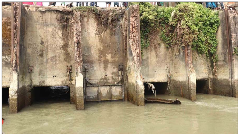
Photo – damaged sluice-gate in Charfession Upazila
